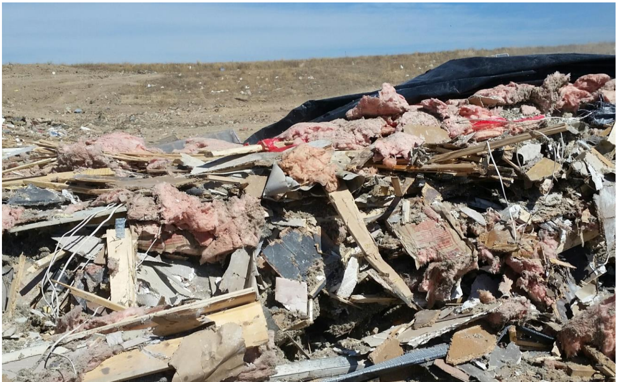
A commercial contractor delivers a prime example of materials identified as C&D. The payload appears to be primarily generated by a knock-down type of demolition process whereby most of the materials; wood, drywall, and fiberglass insulation are broken into small pieces.
